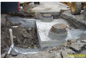
Grease Interceptor- surface views
